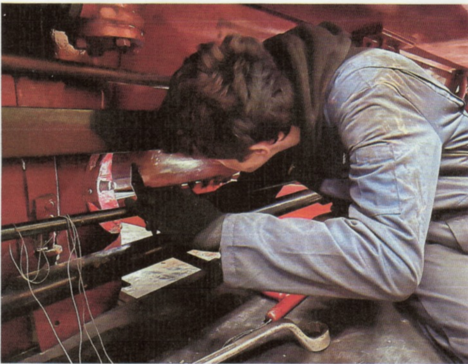
Hands on: Benjamin fits a mudhole door and checks alignment. DAVID GRINDLEY
